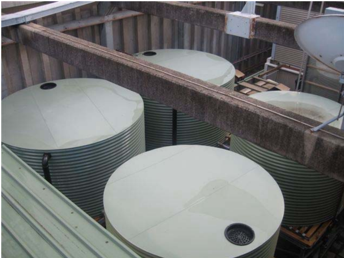
Water tanks installed as part of the Parliament's water harvesting/recycling project
