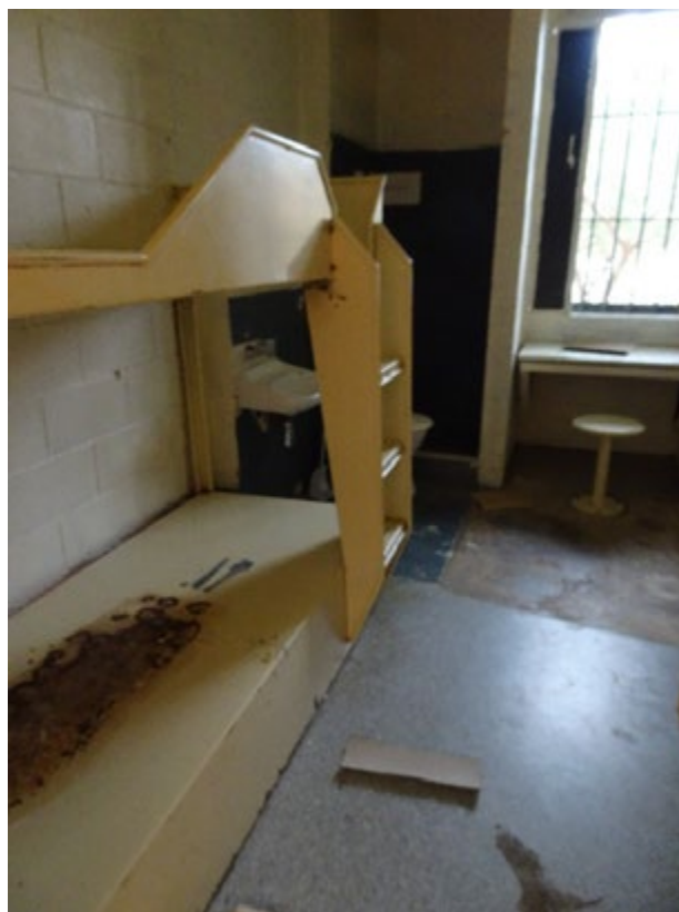
Unused cell, Unit 3B
