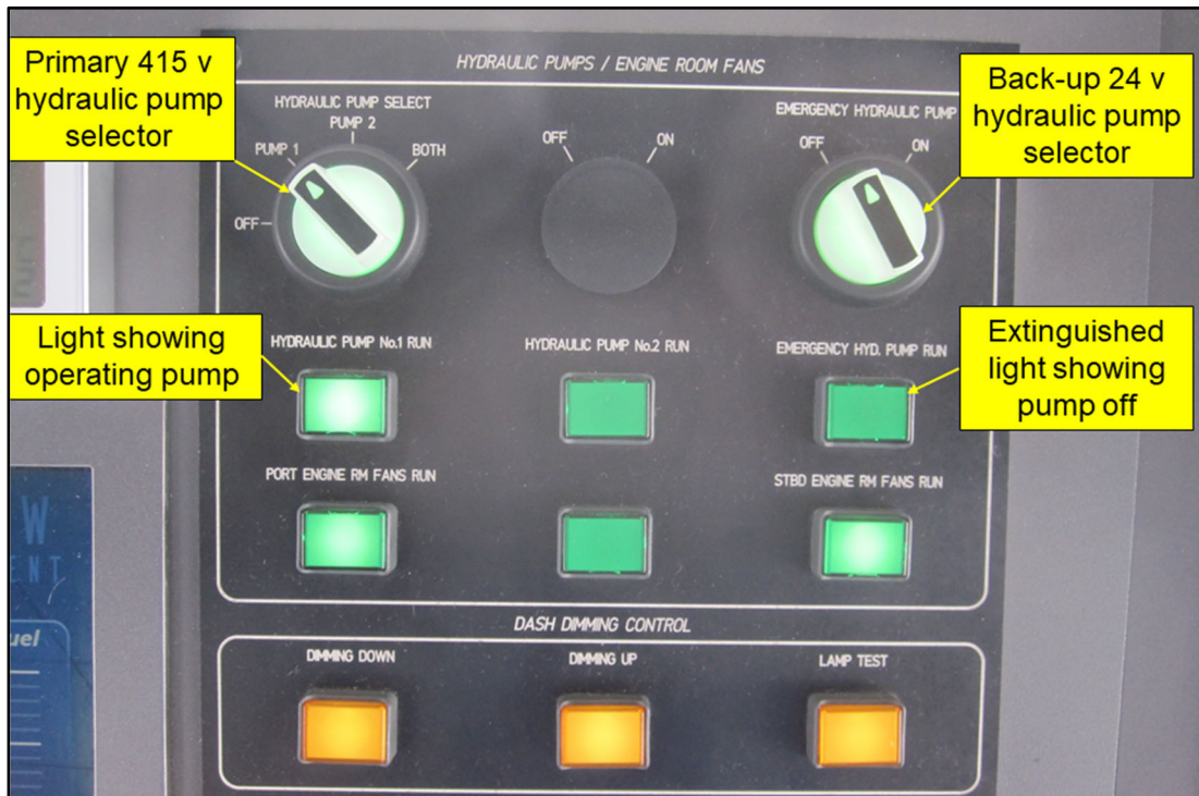
Figure 10: Steering power supply panel in detail
