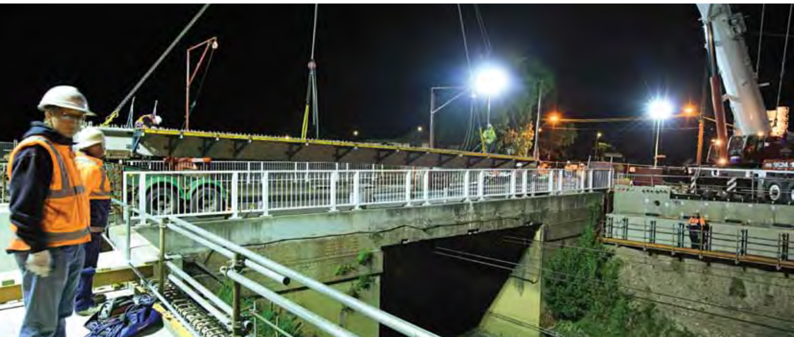
Nightworks on the Kingsgrove to Revesby Quadruplication project, the largest project in the Rail Clearways Program.
