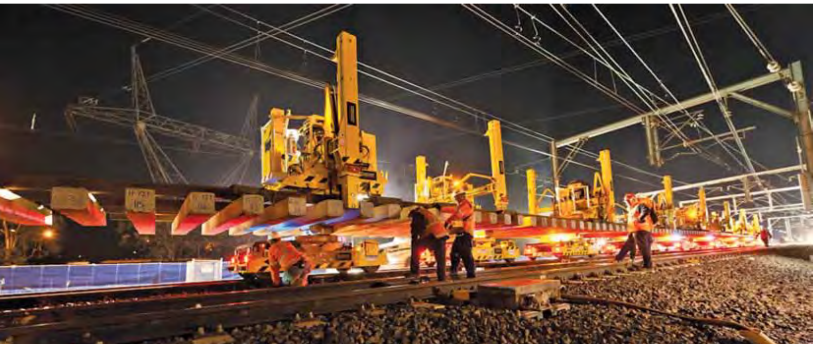
Installing a new track turnout for the South West Rail Link at Glenfield.
