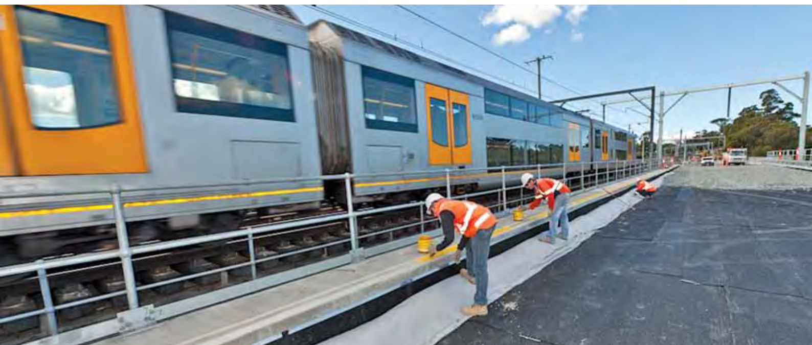
A complex combination of technical, environmental and safety challenges were overcome to complete the works at the Salt Pan Creek.
