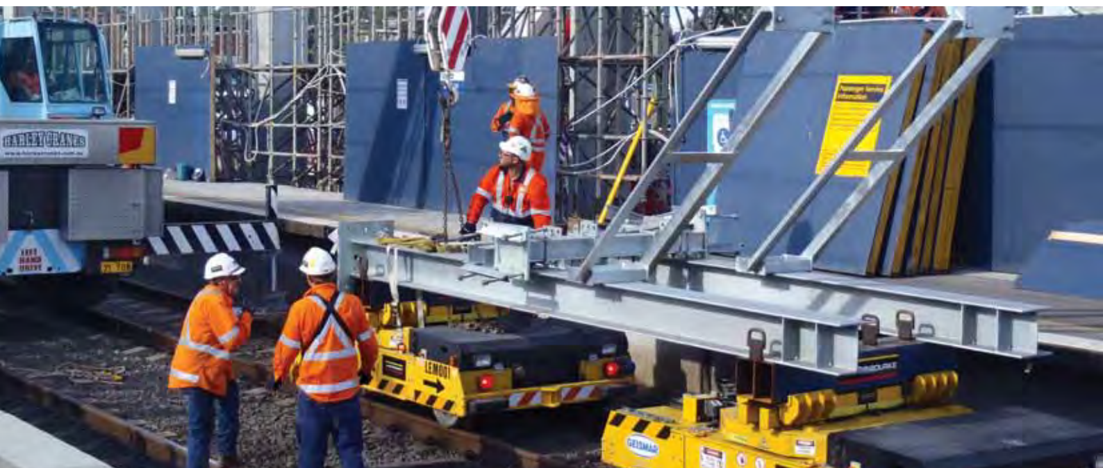
Audits, inspections and reviews verify compliance with TCA's Safety Management System at the Glenfield Station works.
