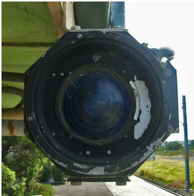
Photo 12: Close up of unlit Guard's indicator at Unanderra Platform
