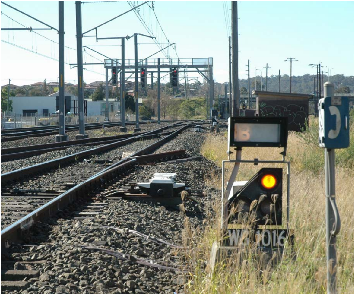
Photo 11: Signal WG1016 showing proceed indication in relation to signal WG1010 at stop
