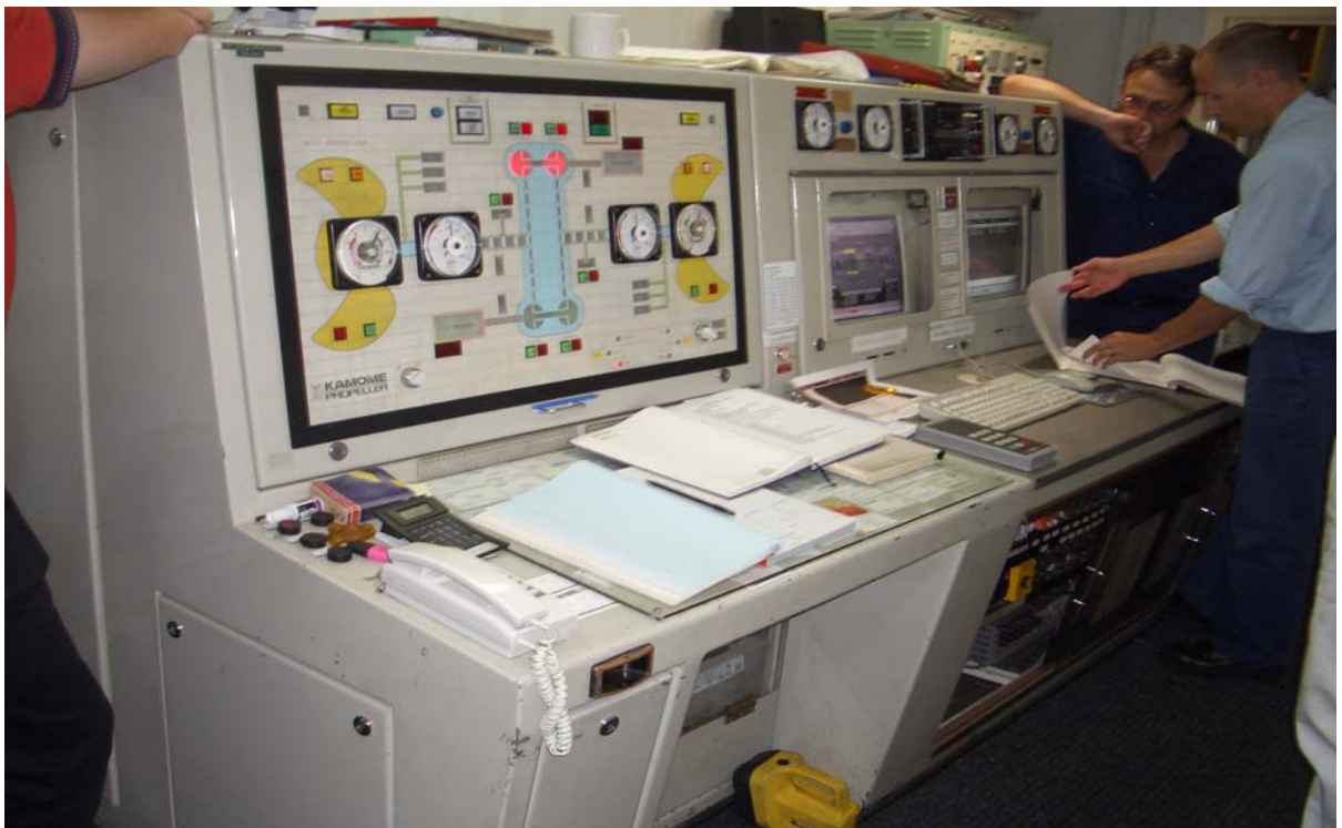
Figure 6: The Machinery Control Room (MCR) Mimic Panel and Data Logger Console
