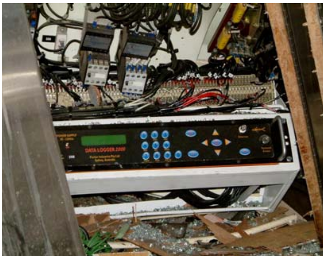
Picture 5: Relatively undamaged data logger in the wreckage of car 6831.
