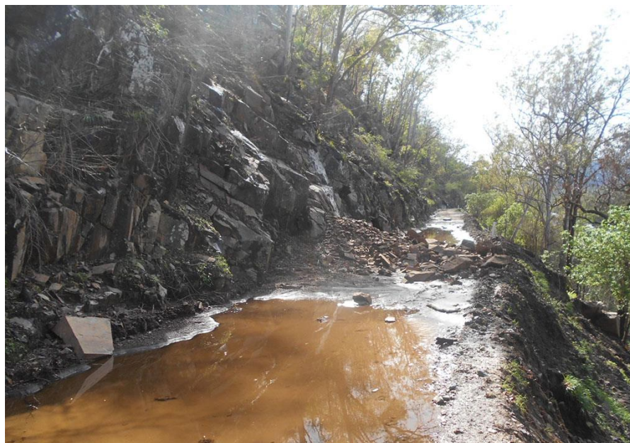
The Kempsey Armidale Road after storm damage in February 2020.
