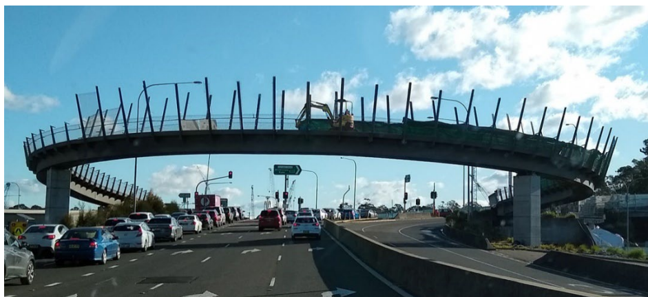
Figure 3: Demolition of Beatrice Bush Bridge during construction of the Rozelle Interchange (source: https://www.groveoz.info/ )
