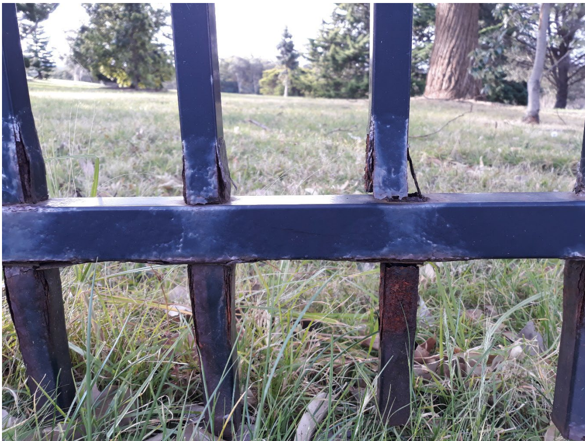
Figure 2: Example of structural failure of a fence panel due to corrosion.
