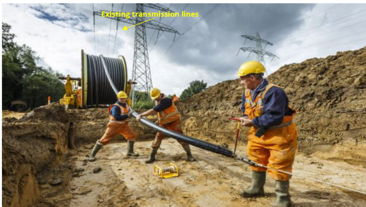
Figure 3. Underground transmission line being installed within existing transmission easement. Source: Renewables Grid Initiative
