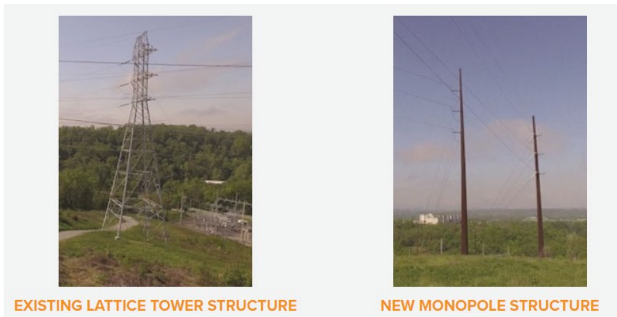
Figure 2: Existing and new transmission structure for the Brunot island-crescent transmission reliability project
