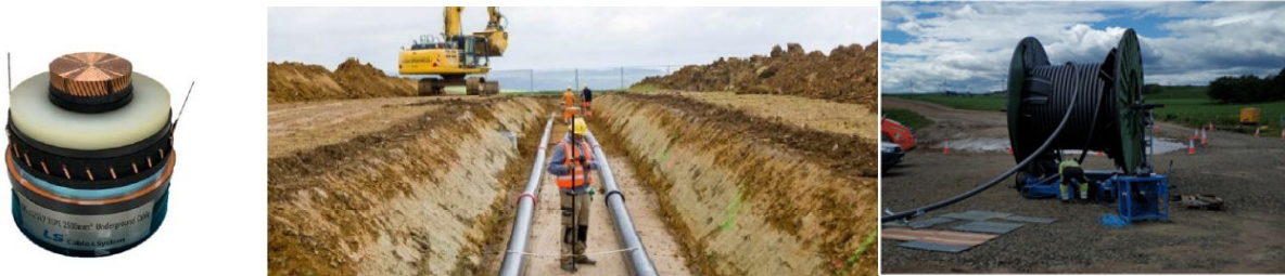
Figure 3: Underground cable infrastructure 6
