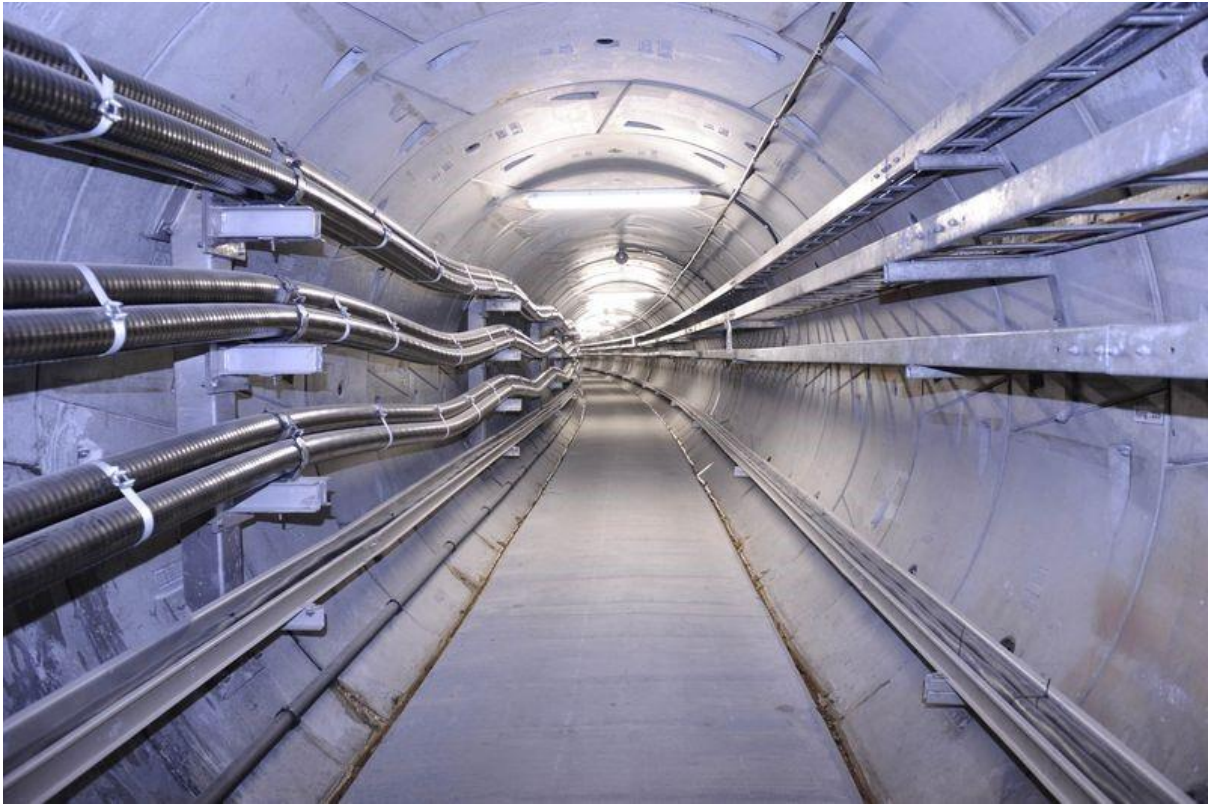
Figure 2 - Ausgrid's 132kV City West cable tunnel
