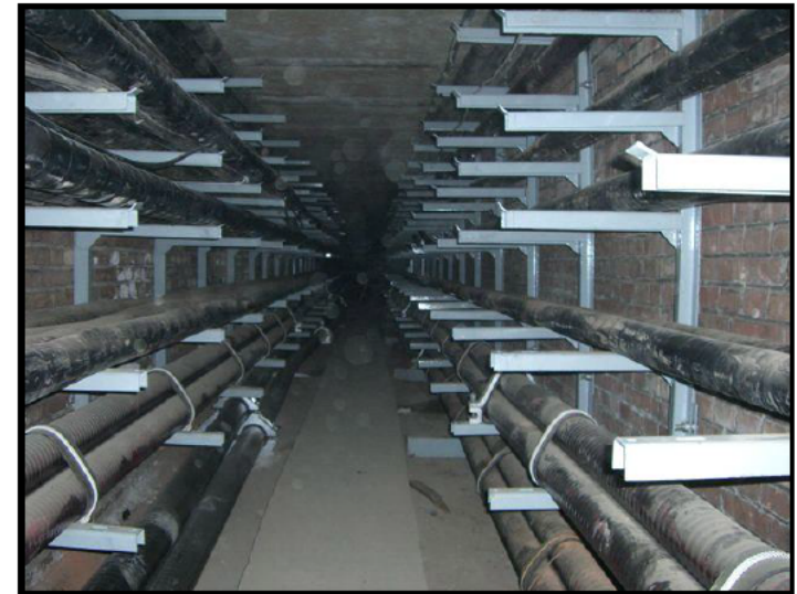
Cable tunnel in Beijing
