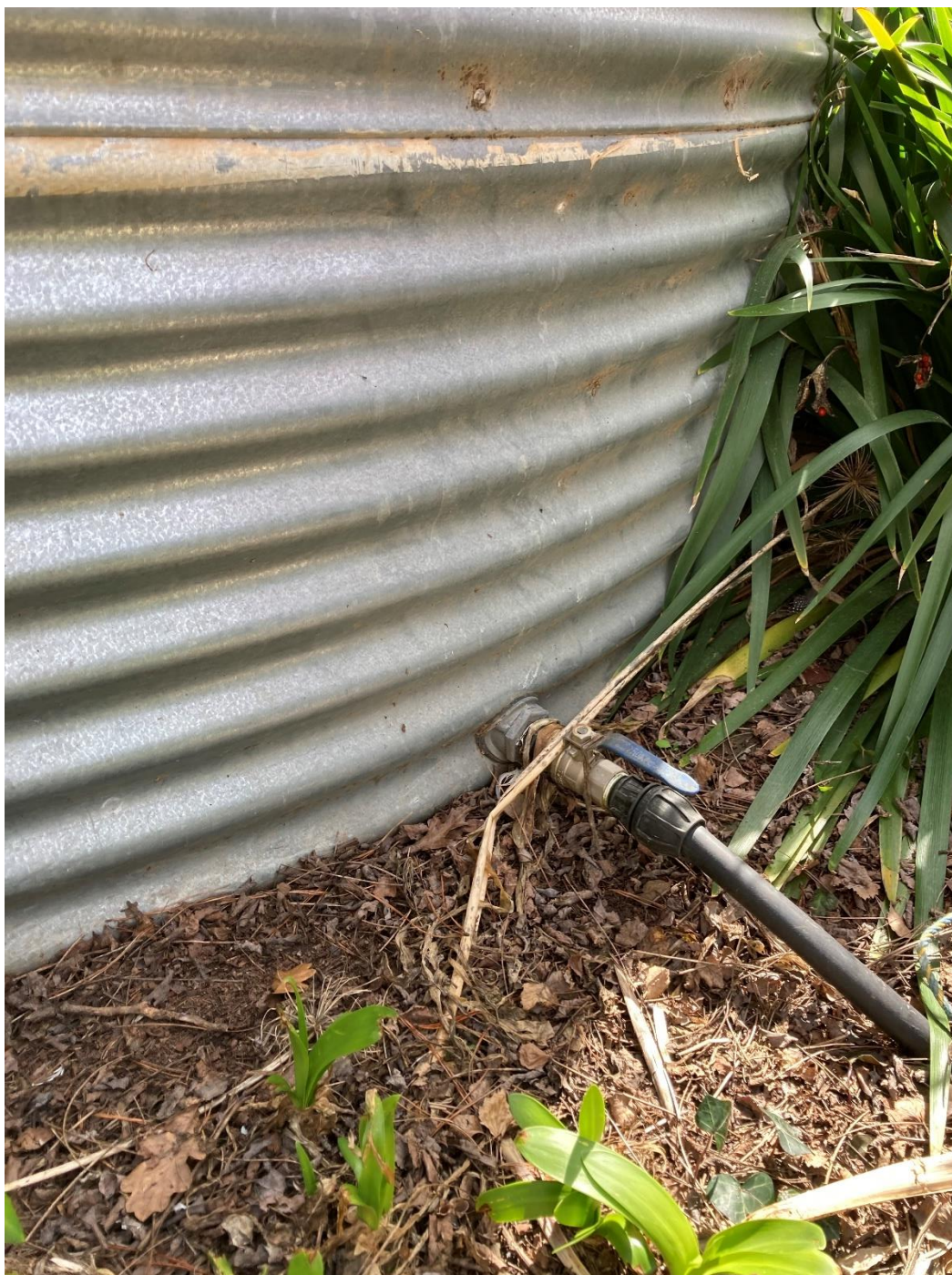
Figure 6. Most water tanks access water from the lower section of water tanks. Water quality at this 'layer' is critical for household water quality.
