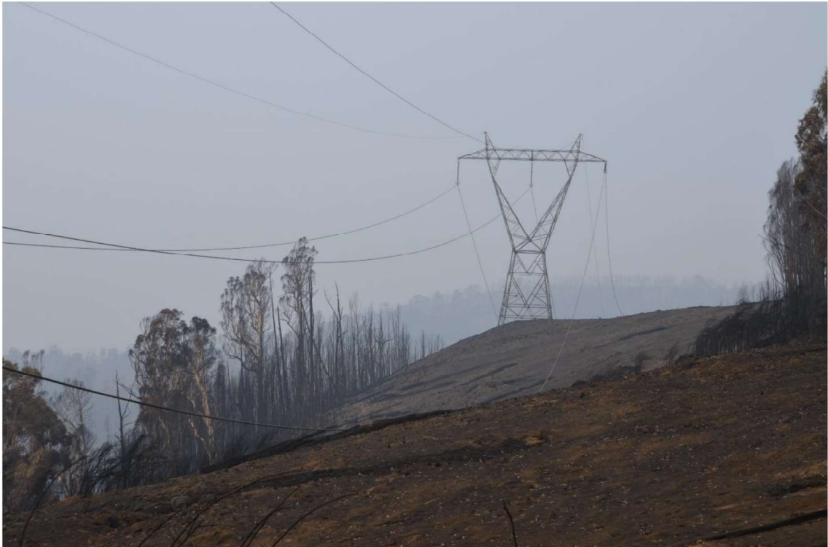
Figure 9 – Line U3 Dropped conductor on ground
