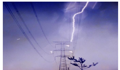
A pair of conductors that do not carry electricity sit at the top of each pylon. When lightning strikes the pylon, the lightning will flow through these conductors harmlessly into the ground, without interfering with the electricity carried by the main conductors.
