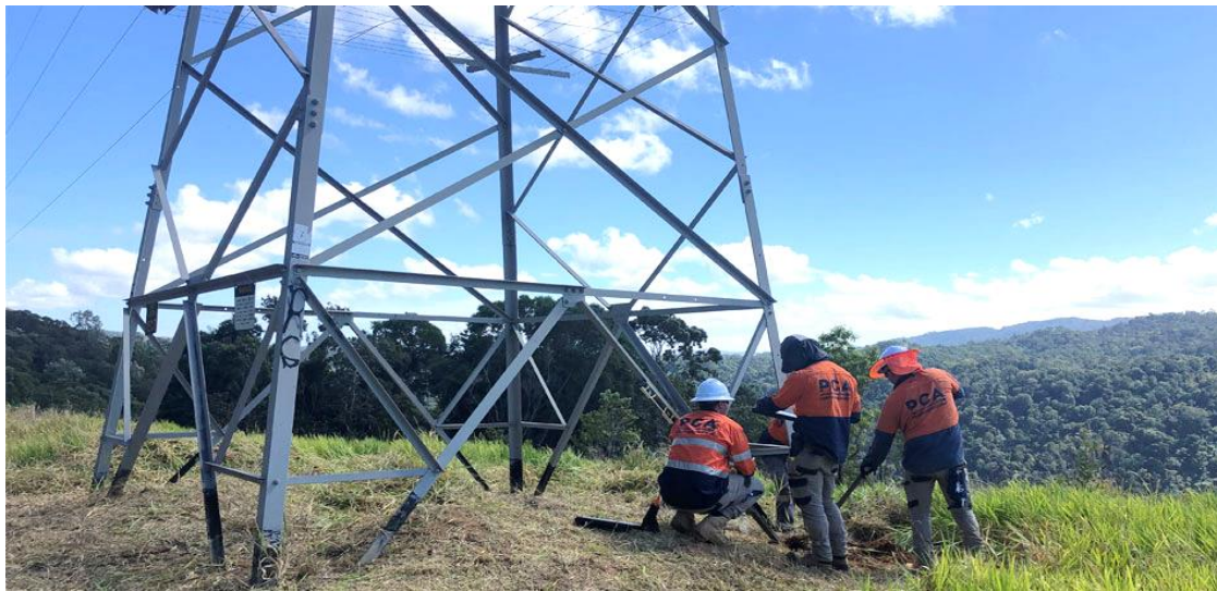
(One of the transmission line towers linking up to the Mt Emerald Wind Farm.)
