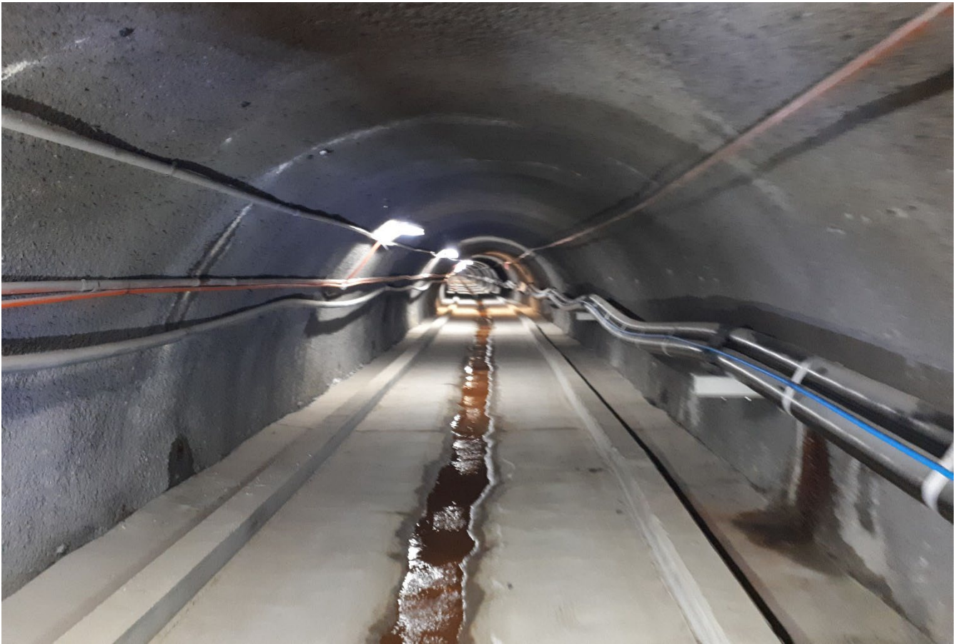
Figure 3 Haymarket Substation tunnel - 330kV cables on the right
