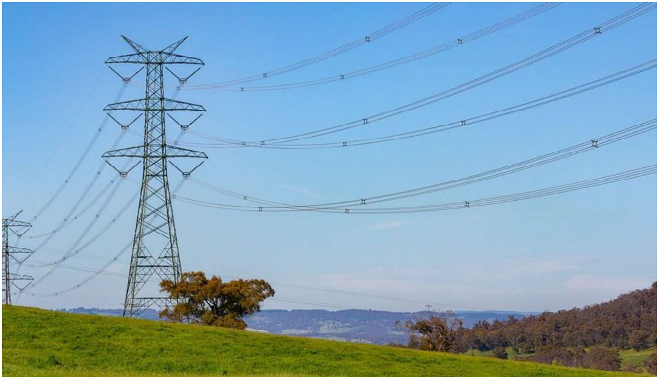
Above: Photo of typical existing transmission line corridor in Snowy Valleys Local Government Area.
