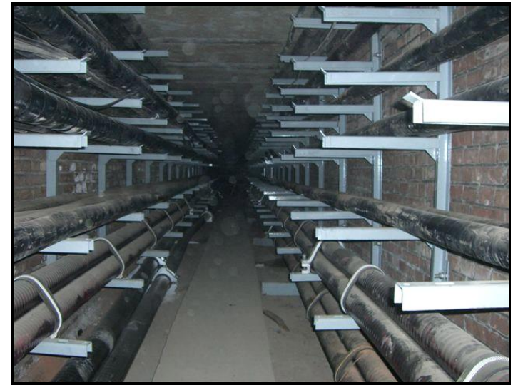
Cable tunnel in Beijing
