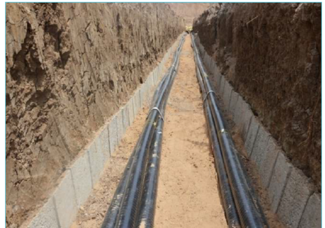
Underground HVDC Trench
