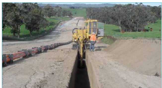
Underground transmission, rather than overhead, at the request of communities and landowners.
