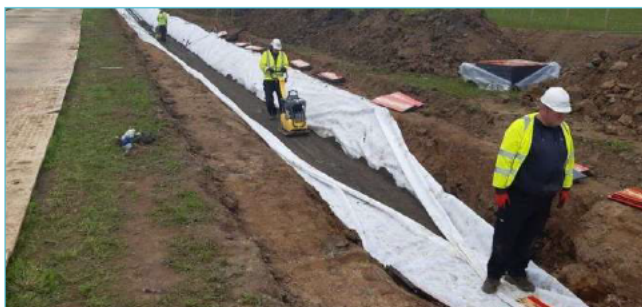
Underground HVDC Trench
