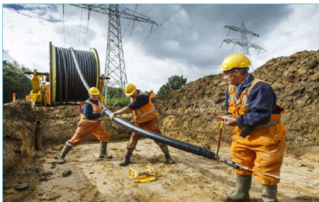
Installation following Basslink – an existing, high voltage overhead transmission line
