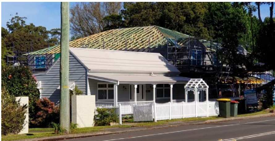
44 Queen Street Berry, overwhelmed by height, bulk and scale of the new 2 storey dual occupancy under construction in Berry’s main street.
