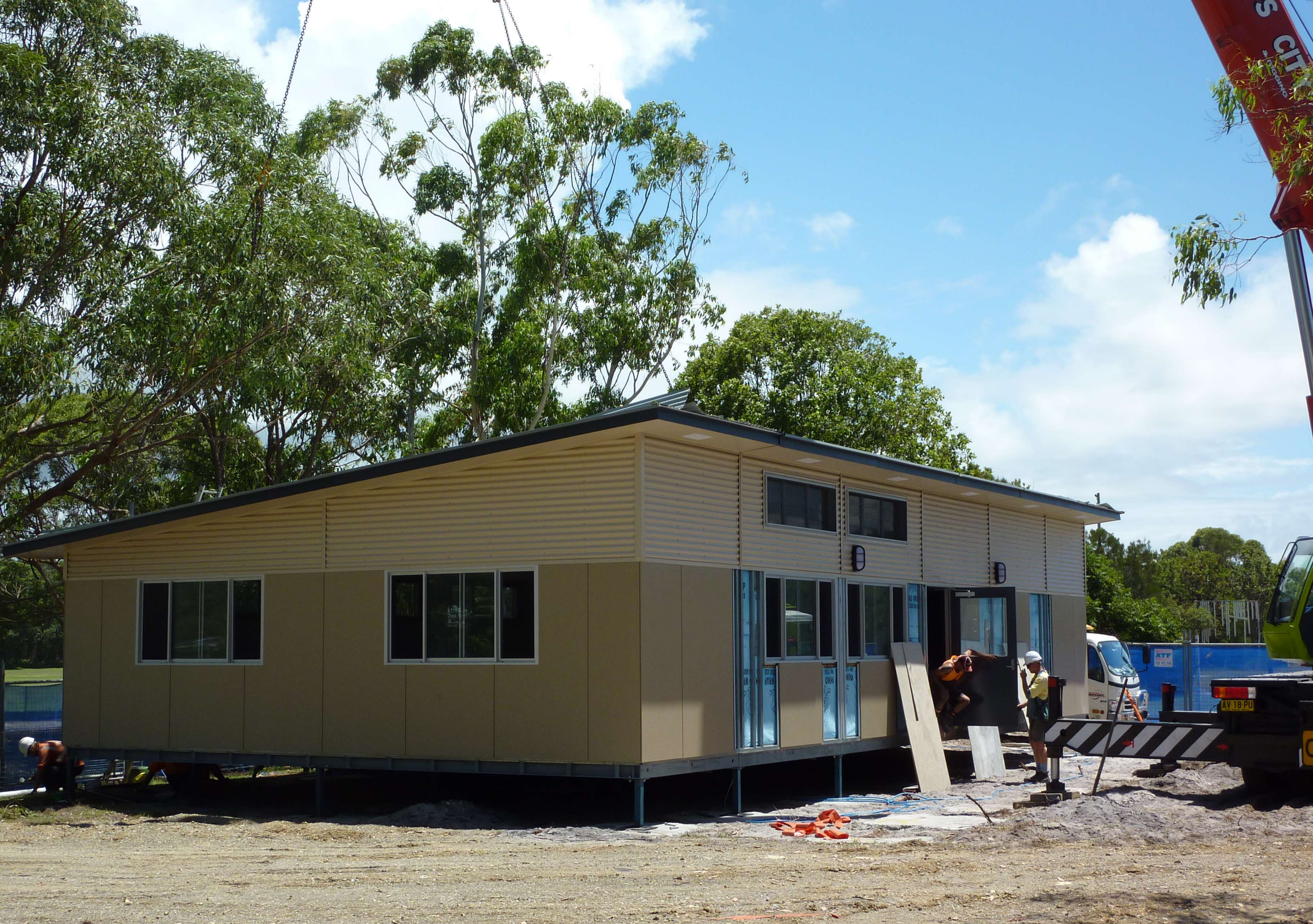
Photo of the building taken in the first week of March - the building is currently still under construction some 10 weeks later.
