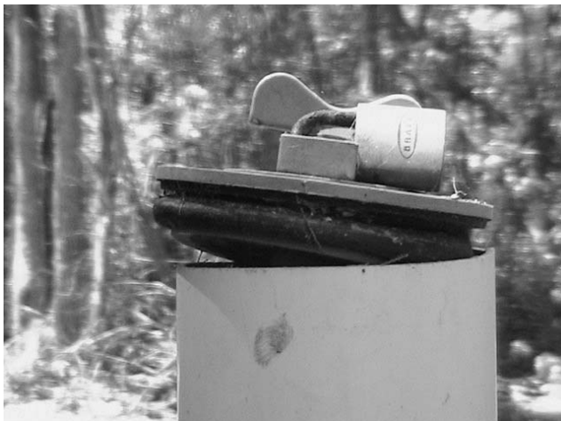
Ineffective locked piezometer
