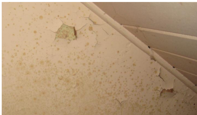
Image 1 - A mould infested ceiling in a public housing property in Millers Point
