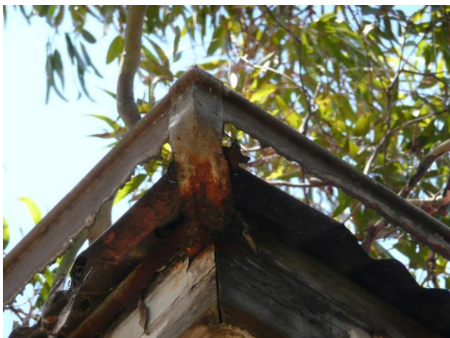
Image 3: Guttering on a public housing property in Copeland St, Erskineville, that had been completely non-functional for at least two years at the time of writing.
