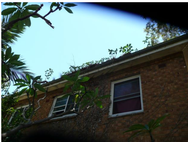
Image 4: Gutters blocked by the presence of plants, Copeland St, Erskineville.
