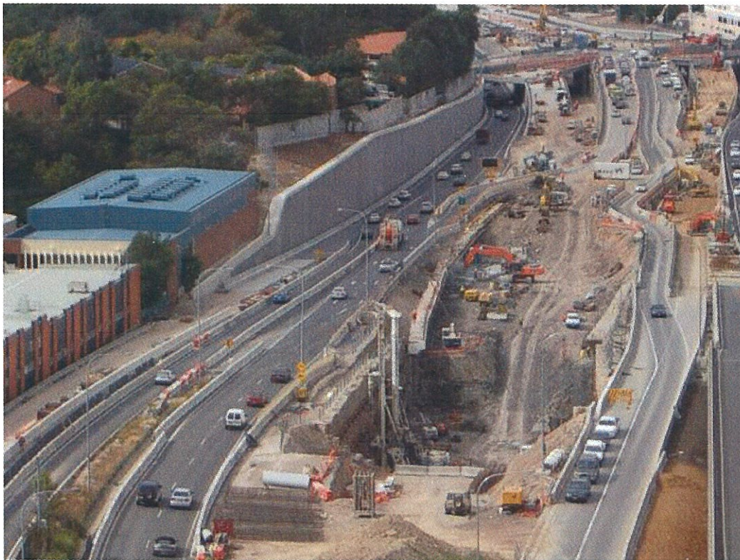
Gore Hill Freeway construction works showing cut and cover entrance/exit to the eastern end of the Lane Cove Tunnel in the foreground and the Reserve Road ramps reconfiguration underway in the background.
