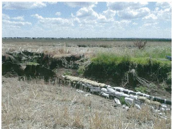
Figure 5: Pipeline induced erosion near Coolah, NSW
