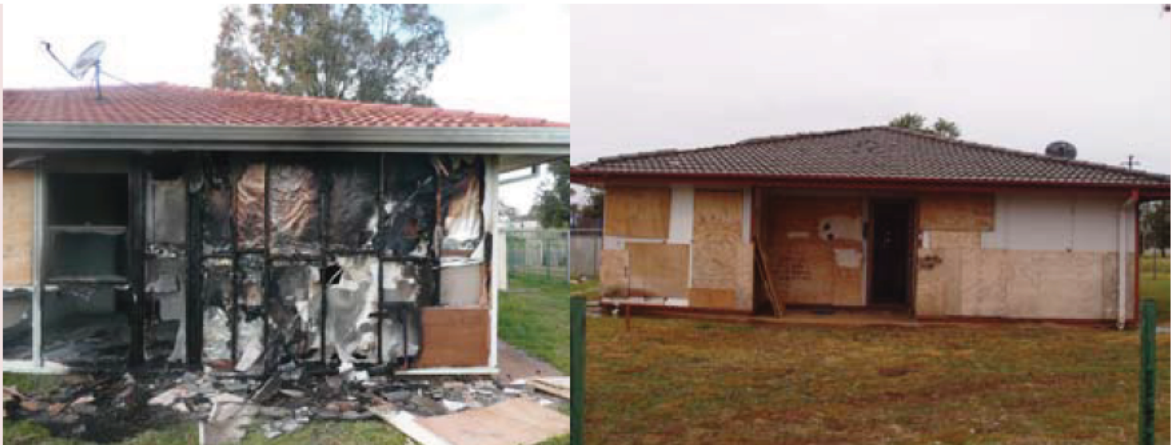
Vandalised properties in Gordon Estate before implementation of Transformation Strategy
