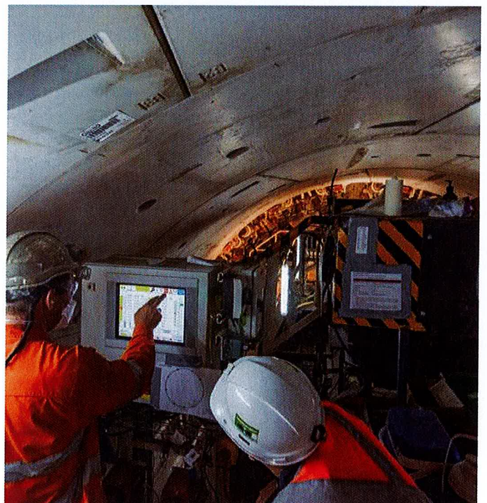
Inside a tunnel boring machine (TBM).
