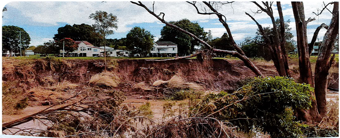
Major riverbank erosion at Casino
