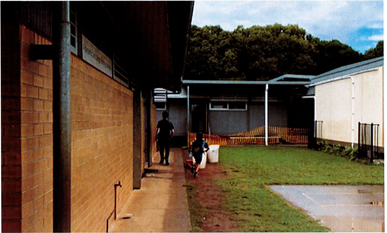
One sheltered walkway from school hall to portable classroom cluster. Shelter ineffective during heavy rain.
