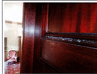
Photo 5: LC Chamber, horizontal surfaces prior to remediation works
