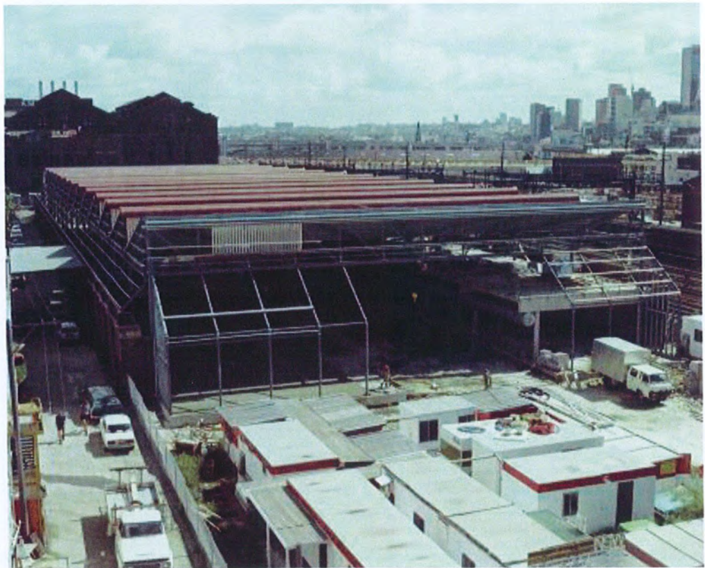
The former 1899 Ultimo Tram Depot under construction for the Powerhouse Museum project. It opened in 1981 as Stage 1 of the Museum with a preview exhibition showing highlights of the collection.
