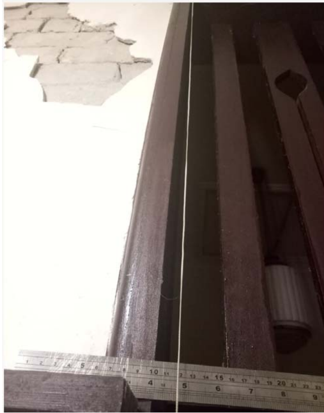
Figure 2 Hallway of No 8 identifying warped doorways
