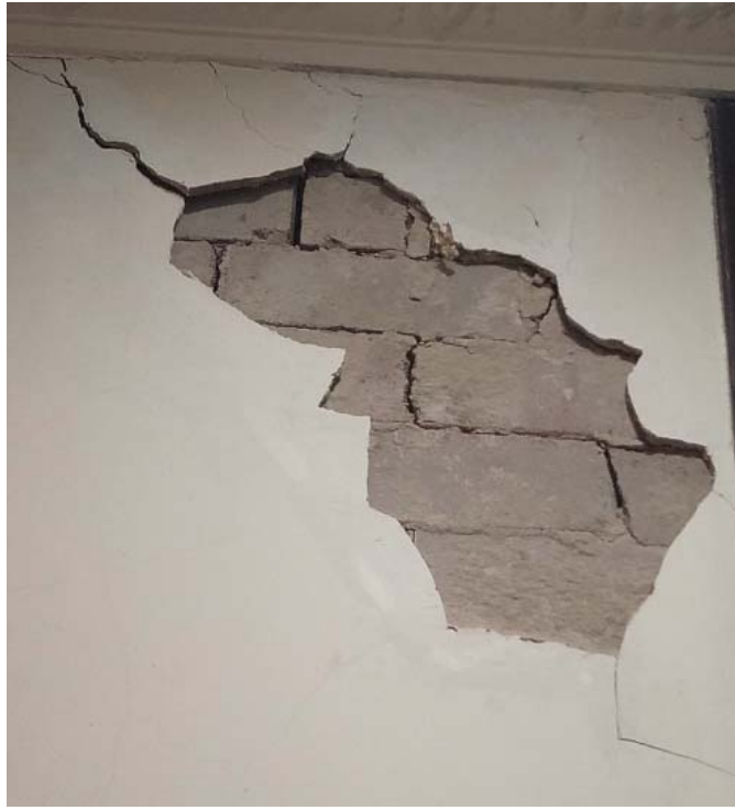
Figure 1 Hallway of No 8 identifying induced strain on internal brickwork
