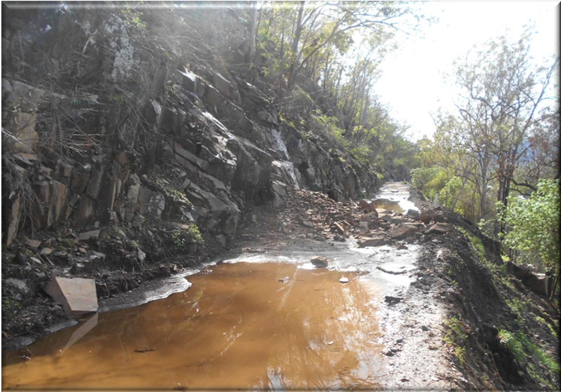
The Kempsey Armidale Road after bushfire and storm damage, late 2019/early 2020.
