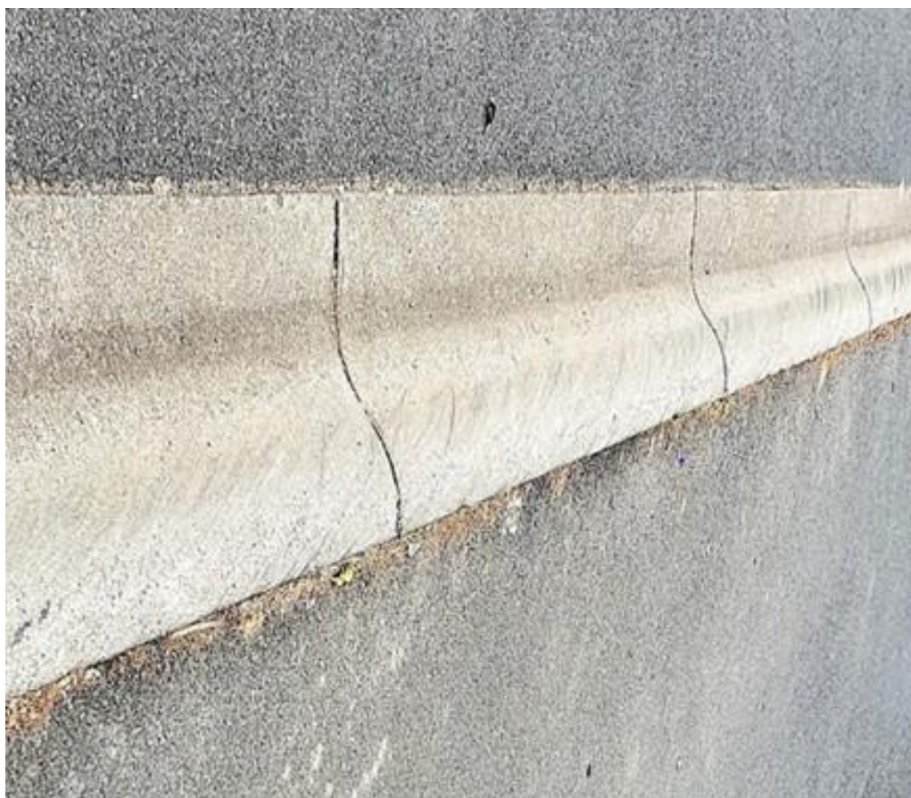
Photo 2: Evidence of vehicles bottoming out on the kerbing
