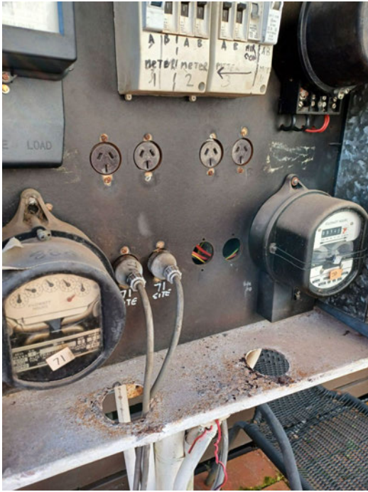
Switchboard and meters
