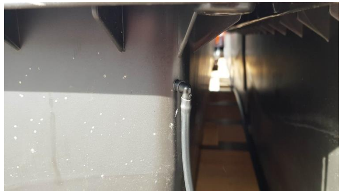
Figure 6: Integrated irrigation system. Cladding is then used to
