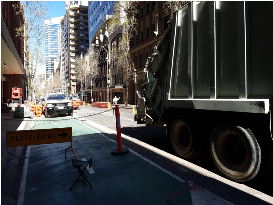
Construction transport management Kent St, Sydney. Road traffic continues. Garbage truck blocking pedestrian detour, with lack of traffic control crossing assistance and corresponding accessibility ramps. Bi-directional cycleway closed with no detour provided (on 1 way street).
