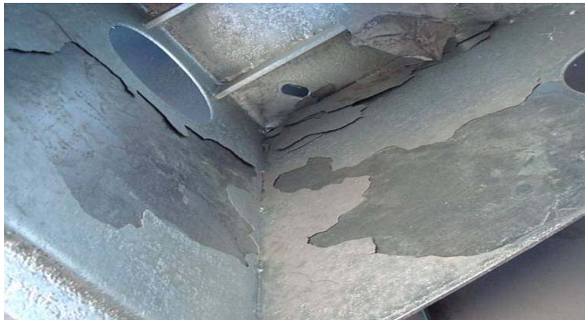
Photo 2 Poor galvanizing due to steel chemistry
