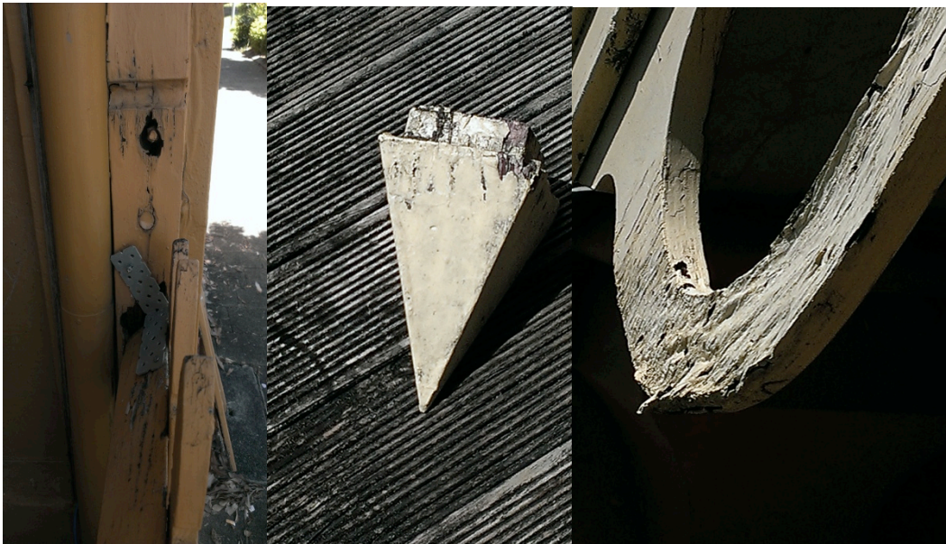
Fencing rotted, fallen and rotten decorative eaves
