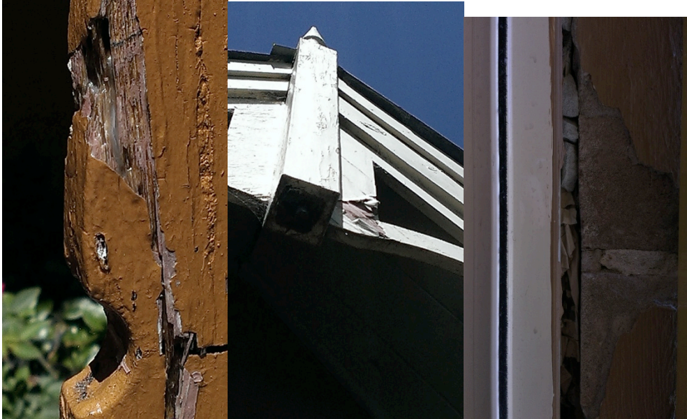
rotten wood, fallen eaves and crumbling masonry
