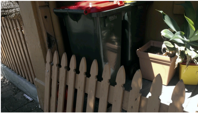
Fence detached from rotten frame
