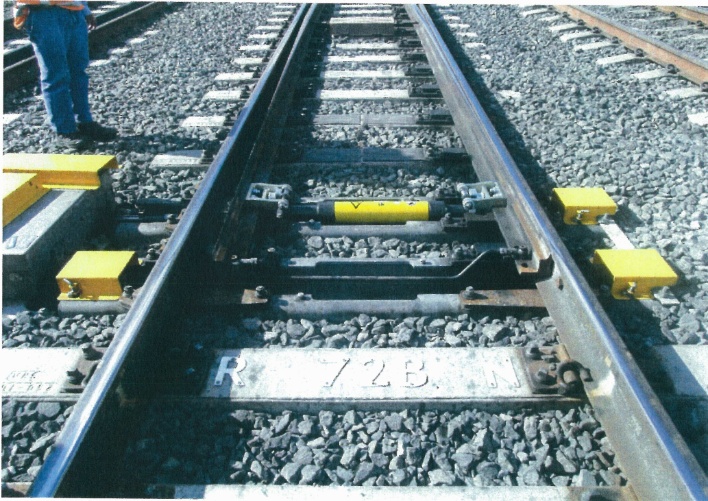
Cover Photo: Spherolock Trial at Campbelltown nearing completion. Planned to replace claw locks in the long term.
