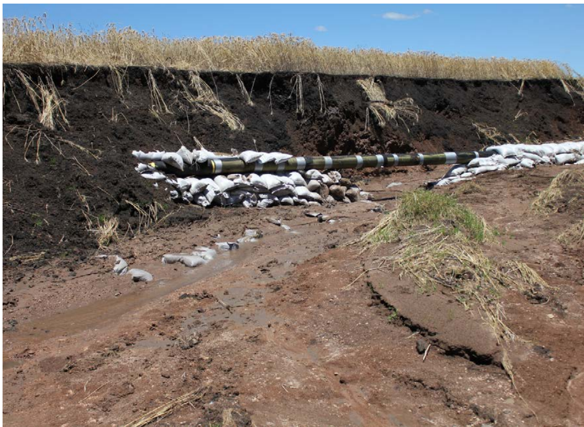
Existing Central Ranges Pipeline exposed to a depth of more than two metres on local floodplain.
