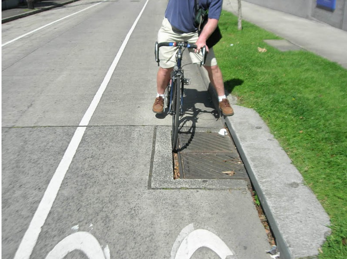
Drainage grate in Balmain show the hazards associated with this type of infrastructure. Photo: Robert Moore Photo: Robert Moore
