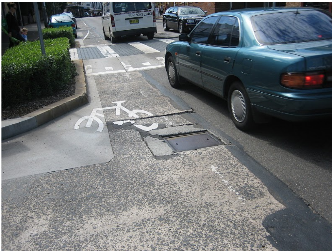
This sunken access plate and uneven surface on a bicycle lane in Balmain can be hazardous to bicycle riders and are difficult to see at night. Photo: Robert Moore
