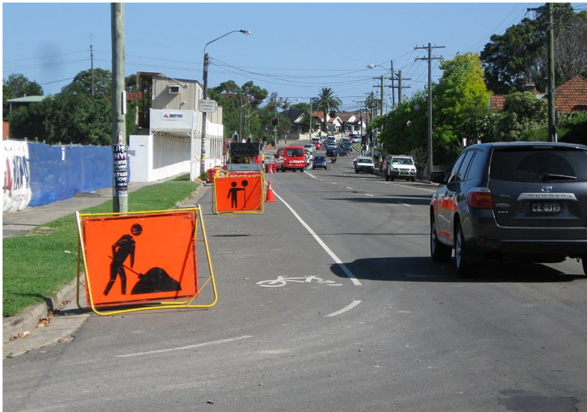
Construction works block bicycle shoulder in Lilyfield. No bicycle detour, warning signs or lower speed restrictions provided. Photo: Robert Moore
