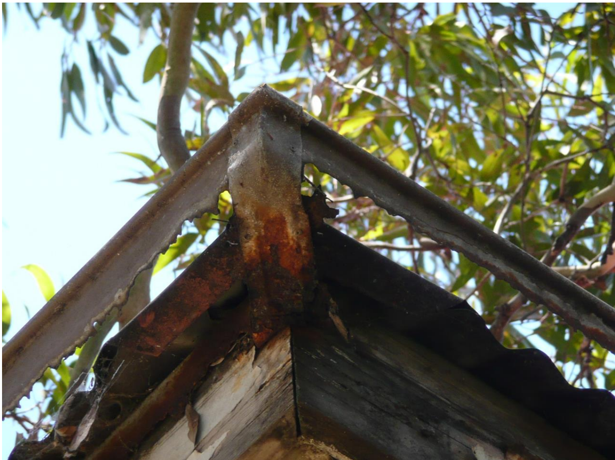
Photo of gutter from Copeland St, Erskineville Housing NSW property
