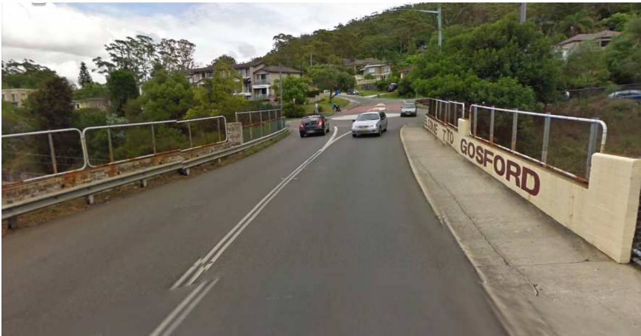
Donnison Street rail overbridge looking west showing inadequate footway/cyclist /traffic areas
